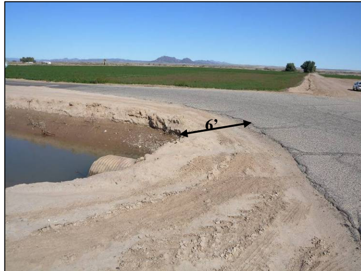
Figure 18: Irrigation Ditch is 6 Feet from Edge of Road in Turning Radius
