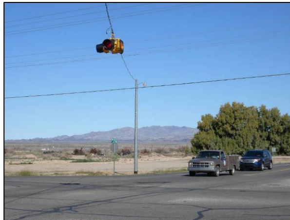
Figure 38: Flashing Beacon at Mohave Road/2 nd Avenue Intersection
