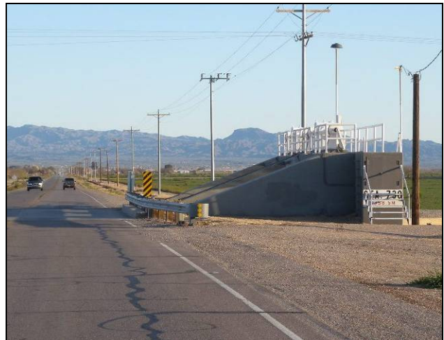
Figure 28: No Barrier to Keep Vehicles from Striking Concrete Structure
