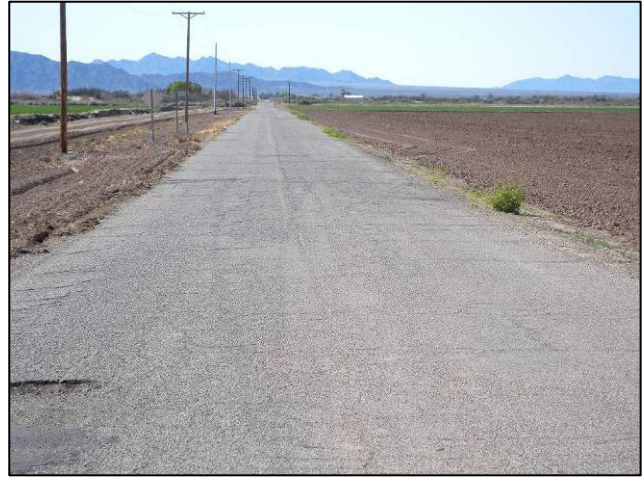
Figure 4: No Pavement Markings on Burns Road
