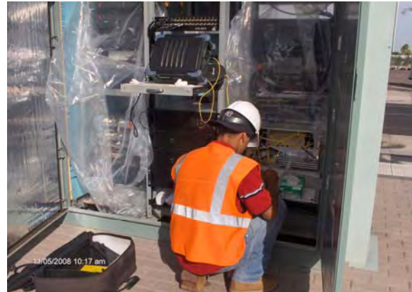
Fiber Testing in Communications Cabinet for Price and Apache Park and Ride Lot
