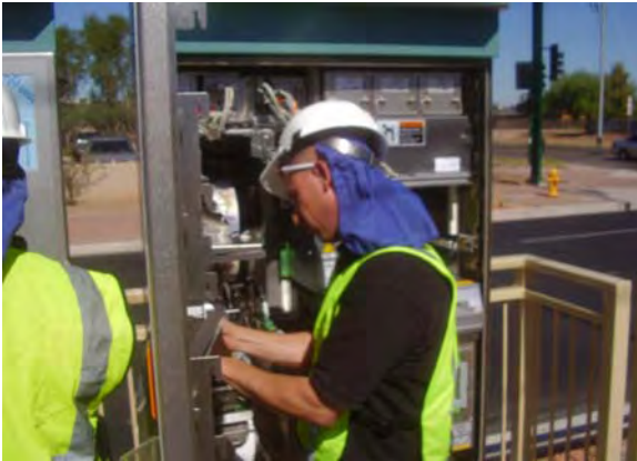
Acceptance Testing at 24 th Street and Washington Station
