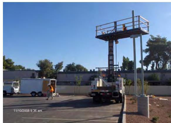
CCTV Camera Installation at 19th Ave and Montebello Park and Ride Lot
