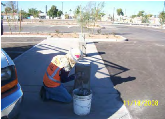
Patching Surface on Motorcycle Bollards 19 th Avenue/Montebello Park and Ride Facility
