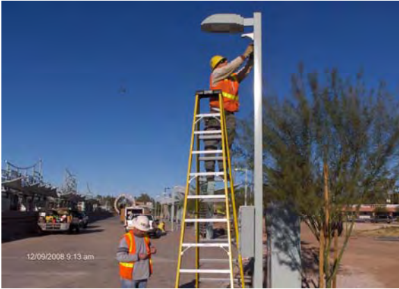
CCTV Camera Installation at Central and Camelback Station Transit Center
