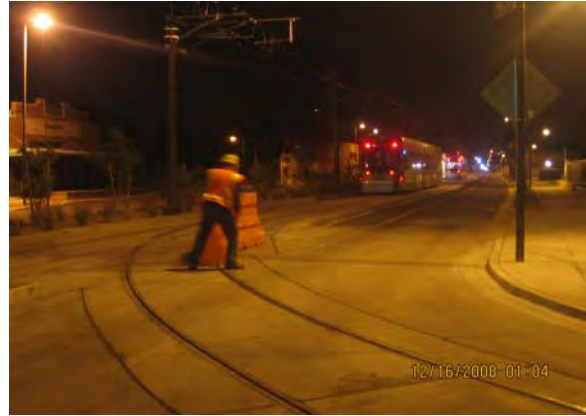
11 th Street Loop Live Wire Test
