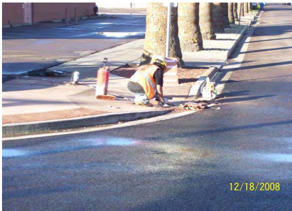
Punch List Ramp Repair
