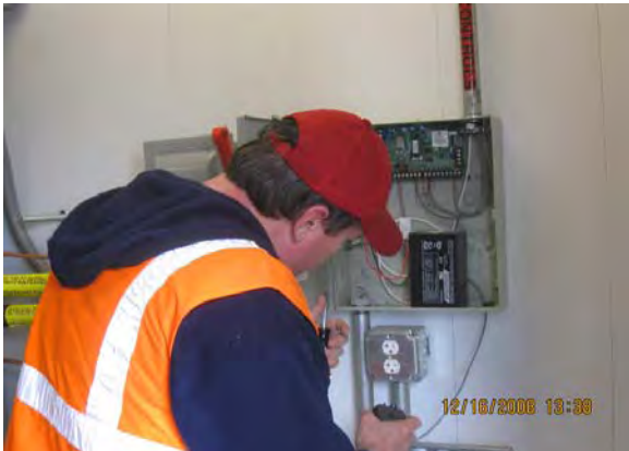
Substation Fire Alarm Test
