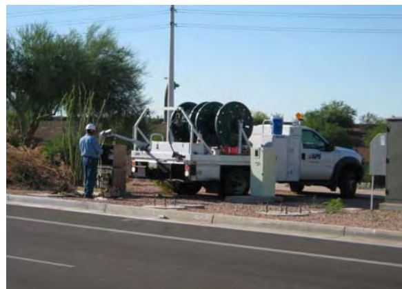
APS onsite preparing TPSS No.3 to be energized
