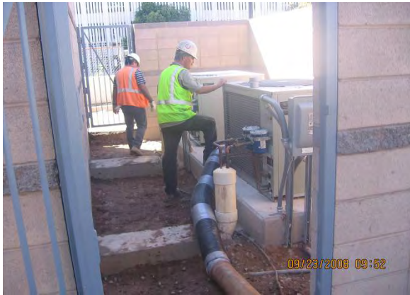
TPSS No. 2 – Removal of Non-compliant Rock
