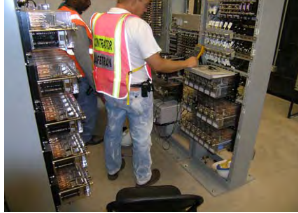
Testing of New Track Transformer Circuits at Sycamore Interlocking
