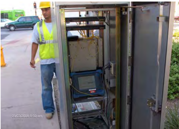
Fiber Splice Testing at Mid Level Switch #2
