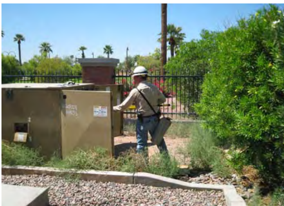
APS onsite preparing TPSS No.3 to be energized
