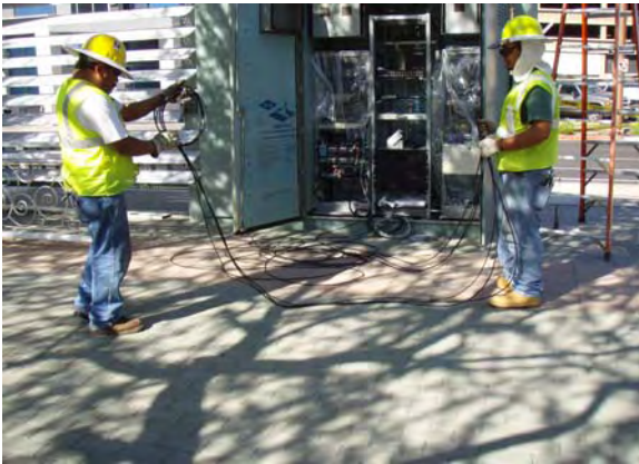
Station Rewiring to Support Fittings Replacement at 1st and Van Buren Station
