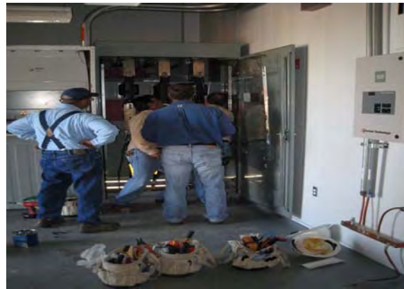
SRP onsite preparing TPSS No.1 to be energized
