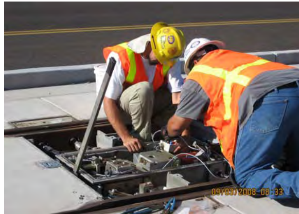
Switch Machine Maintenance at Sycamore Interlocking
