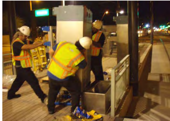
TVM Installation at McClintock and Apache Station
