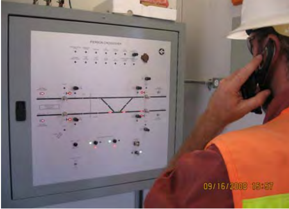
Operational Testing at Montebello Interlocking
