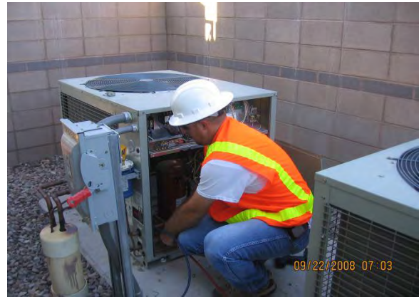
TPSS No. 4 – Testing of HVAC System
