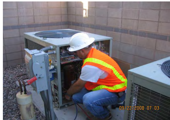
TPSS No. 4 – Testing of HVAC System
