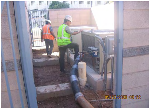
TPSS No. 2 – Removal of Non-compliant Rock
