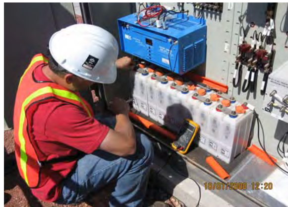
Battery Discharge Test at Dobson Interlocking
