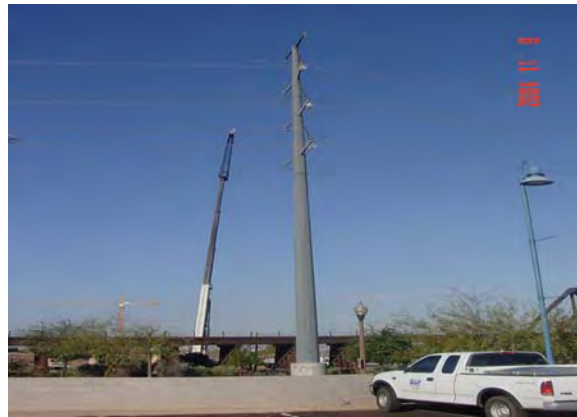
SRP 230 kV over Town Lake Bridge
