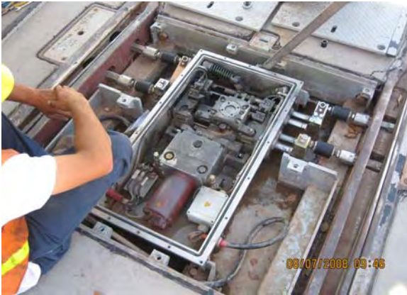
Switch Machine Adjustment at Montebello Interlocking
