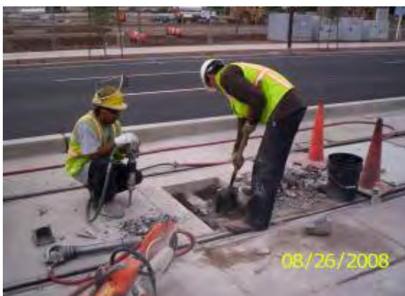
Placement of Surge Arrester at Feeder OCS Poles on 19 th Avenue
