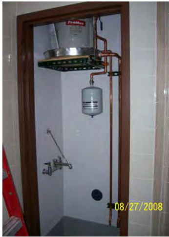
Water Heater Installation 19 th Avenue/Camelback PNR Facility
