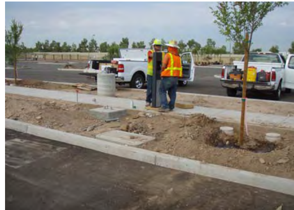
Emergency Telephone Installation at Price Freeway and Apache Park and Ride Lot
