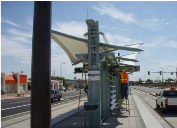
Terminating Device Cable at 19th Avenue and Camelback Station
