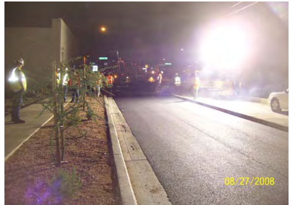
Rubberized AC installation on the slip lane between 16 th and 18 th Streets on Jefferson
