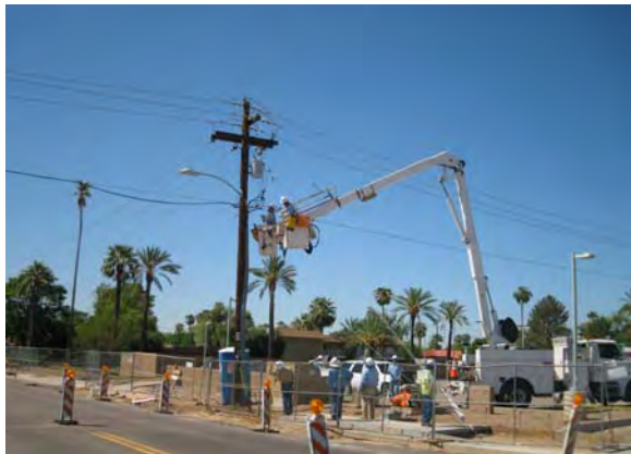
APS removing overhead electric and poles at Central Avenue and Camelback Road Park-and-Ride
