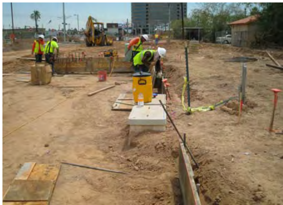
Relocating Junction Boxes at Central Avenue and Camelback Road Park and Ride
