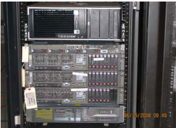
AFCS DCIS Servers in OMC Communications Room
