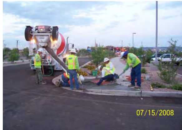
Tactile Warning - Camelback and 19 th Avenue
