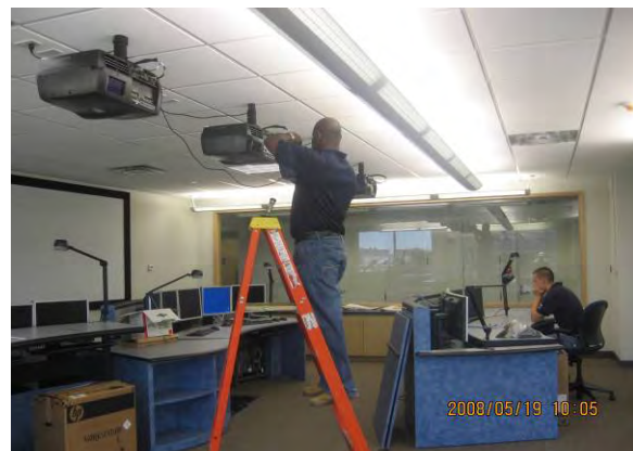
Connecting Overhead Projectors at OCC Operations Room
