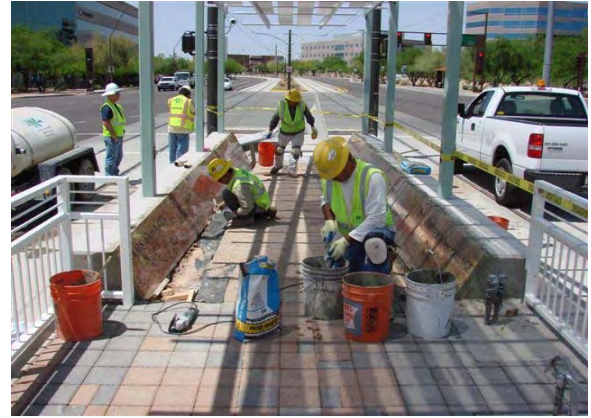
Priest/Washington Station Art Installation
