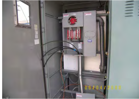
Station at Apache Boulevard and McClintock ready. For SRP to set electric meter
