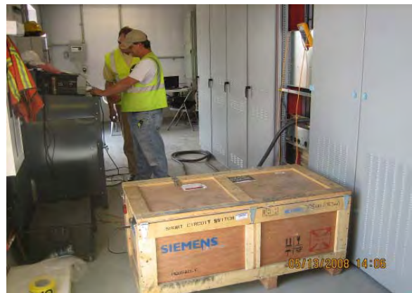
Short Circuit Test in TPSS No. 10
