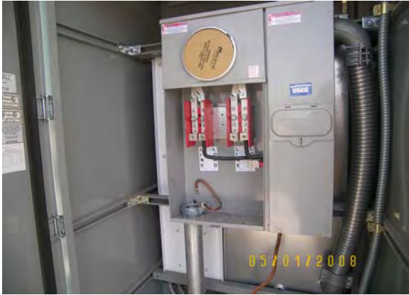
Station at Rural and Tyler – passed Inspection ready for APS to pull cable and set electric meter
