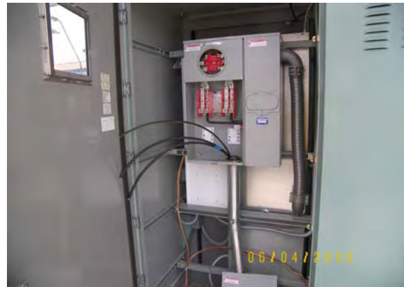
Station at Central Avenue and McDowell Road passed inspection, and energized
