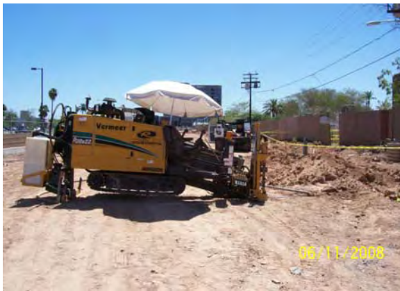
APS Power Conversion - Central and Camelback
