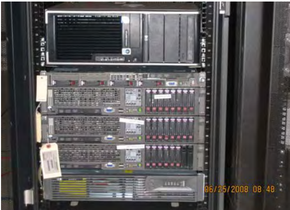
AFCS DCIS Servers in OMC Communications Room
