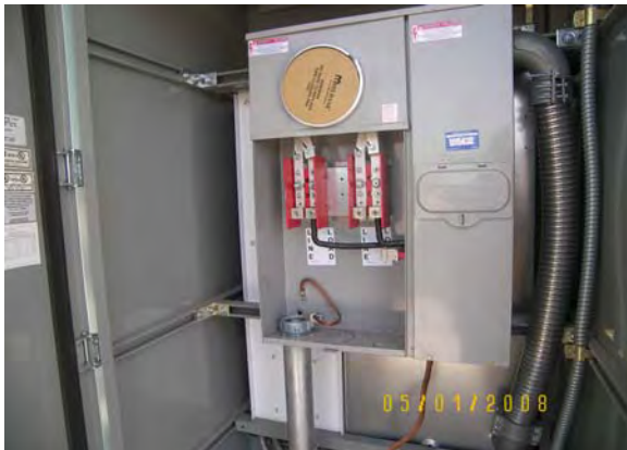
Station at Central Avenue and Indian School Road flat strap placed and ready for inspection.
