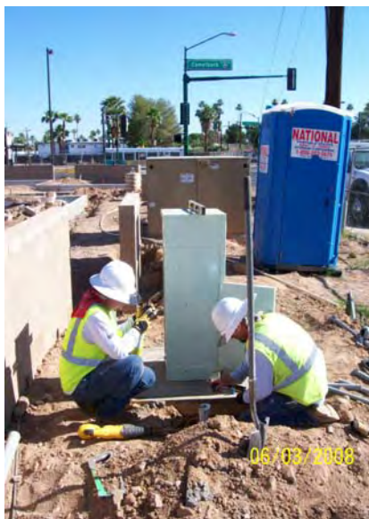
Power Service - Central and Camelback
