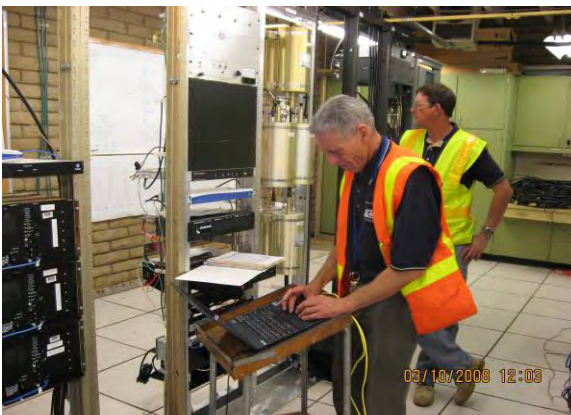
Configuring Data Radio Equipment at South Mountain Radio Site
