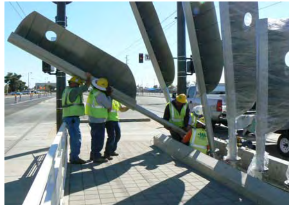
Installation of 38 th Street Station Artwork by Stuart Keeler and Michael Machnic
