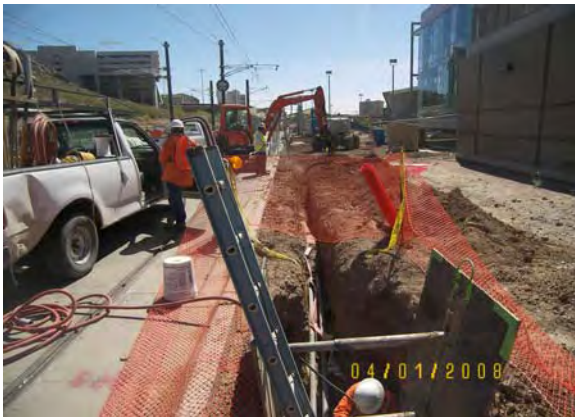
Station at 5 th Street and College - SSW trenching and placing conduits for APS so power can be provide to Station
