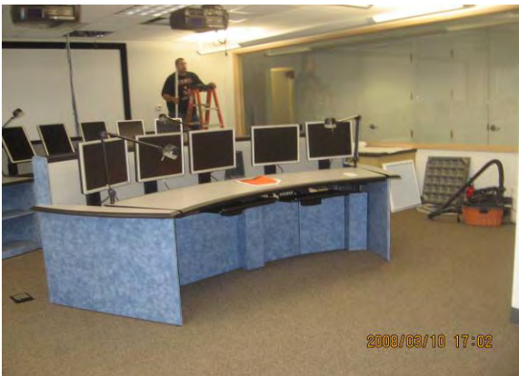
Workstation Consoles and Monitors Setup at OCC Operations Room
