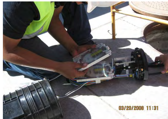
Inspection of Fiber Splice Trays within Fiber Splice Enclosure at LS4
