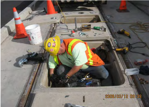
Rail Bonds for Impedance Bonds at Culver Interlocking
