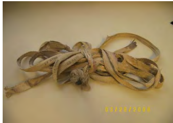
Station at Center Parkway – flat strap that obstructed and was removed from conduit that feed Center Parkway Station
