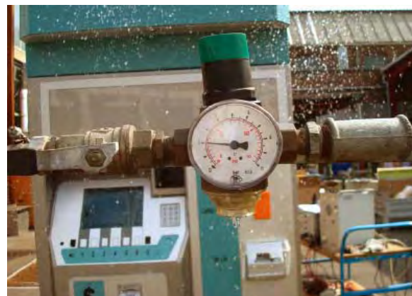
Monitoring Water Flow during Water Spray Test
