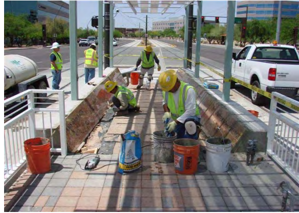
Priest/Washington Station Art Installation
