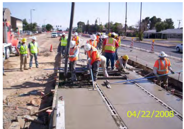
Last Concrete pour for the Guideway on the CP/EV Light Rail Project
