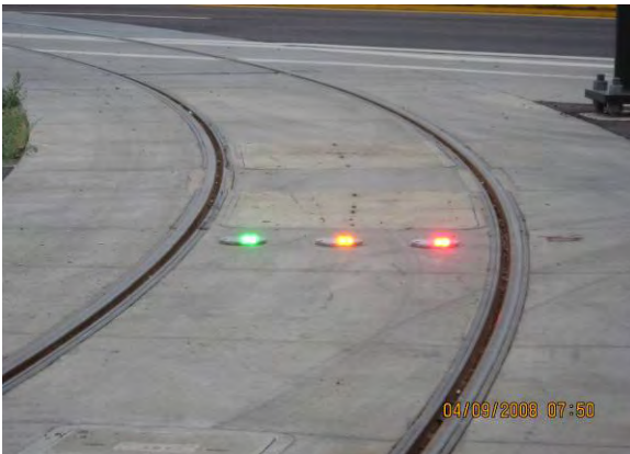
Testing Embedded Signals at Yard Entrance Crossover
