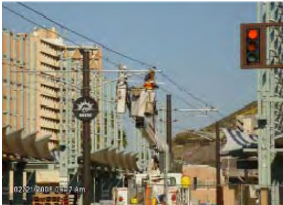
Regulating Wire Runs 45 and 46 (University/Rural Station)
