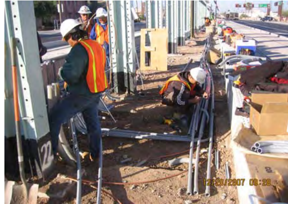
Underground Electrical Installation at Smith Martin and Apache Station
