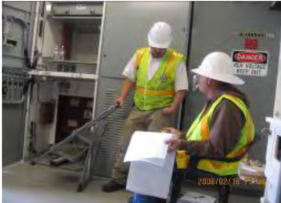
TPSS No. 6 – Siemens Onsite to Perform Precommissioning Tests
