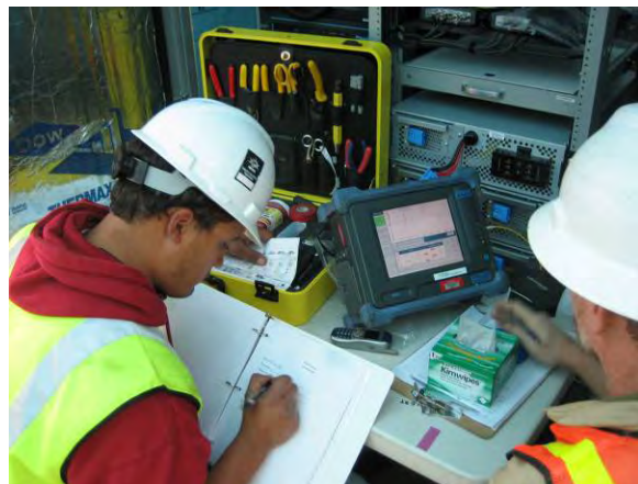
OTDR Testing for CTS backbone Fiber at 5th/College Station
