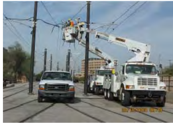
Mill Pocket Track – Regulating OCS
