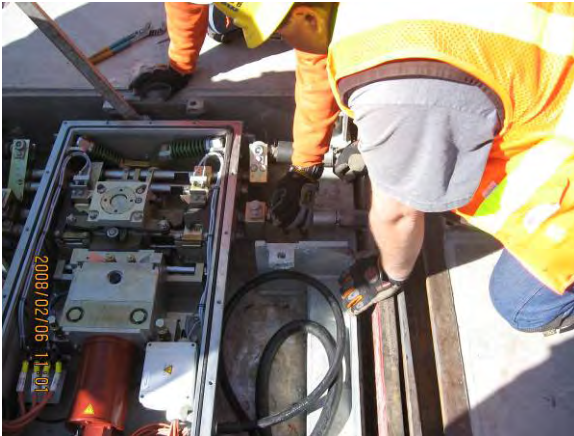
Adjusting Mainline Switch Machines at Dobson Interlocking
