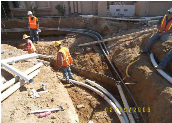
LS1 - SRP Power, Qwest and Cox relocating their facilities which were in conflict with redesign of private irrigation redesign
