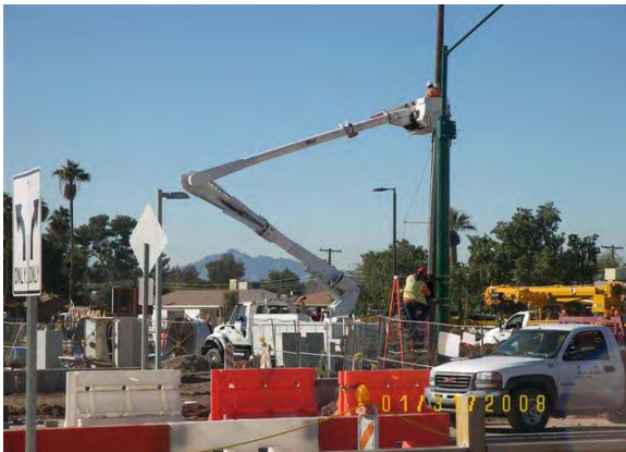
LS1 - SRP Power removing overhead facilities on 19 th Avenue from Missouri Avenue to Bethany Home Road
