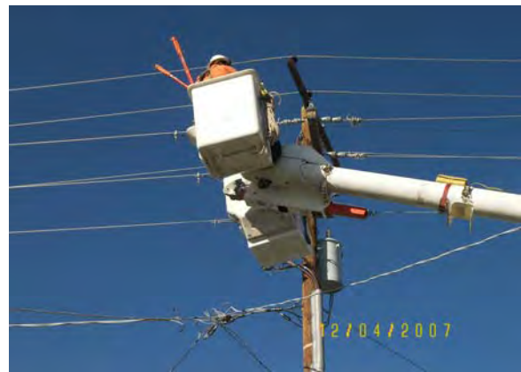
LS1 - SRP Power removing overhead facilities on 19 th Avenue from Georgia to Missouri Avenue
