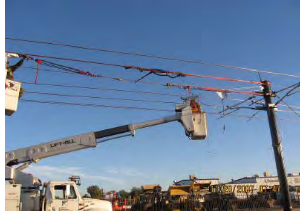
Contact Wire Termination for Wire Run 30
