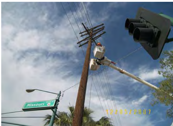
LS1 - SRP Power removing overhead facilities on 19 th Avenue from Georgia to Missouri Avenue
