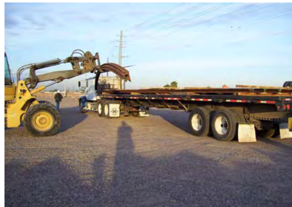
Issuance of Curved Rail for the 11 th Street Interlock to the LS3 Contractor
