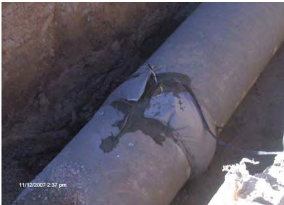
Grouted joint and installed anode with test station lead wires on 48-inch water Line
