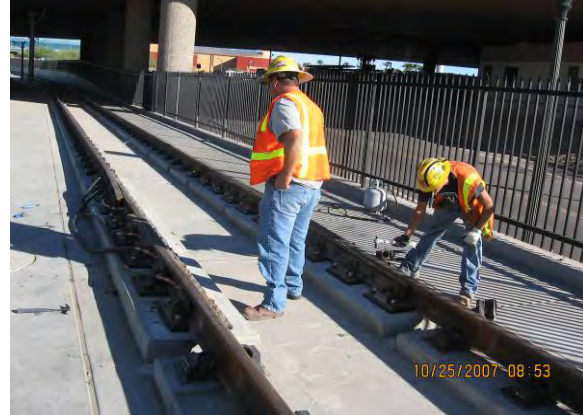
Expansion Joint Rail Bonding at Tempe Town Lake Bridge
