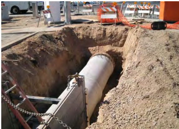
Done - final SRP irrigation pipe connection at Main Street and Sycamore in LS5
