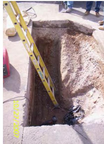
Crews excavated to find the installed Magnesium Anodes for the CP Test Station lead wires on the 12 Water Line tie-in.
