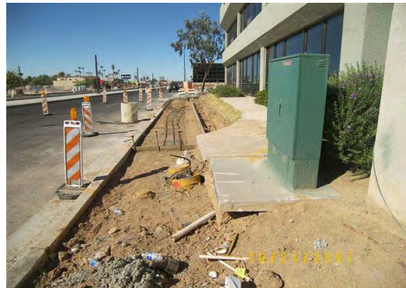
Grade cuts impacting existing utility infrastructures along Camelback Road in LS1
