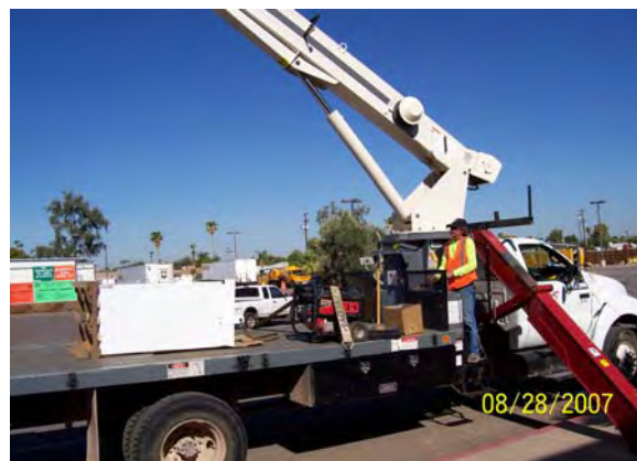
Traffic Controller Cabinet being issued to the LS5 Contractor
