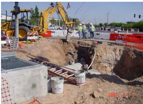
SRP-Irrigation installing new irrigation structure at Main Street and Dobson Road in LS5
