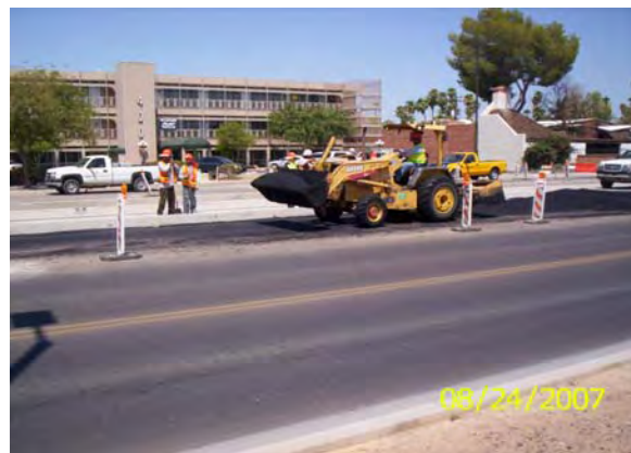
AC Paving - Crews placing AC in the strip area on Camelback Road near 3rd Avenue.
