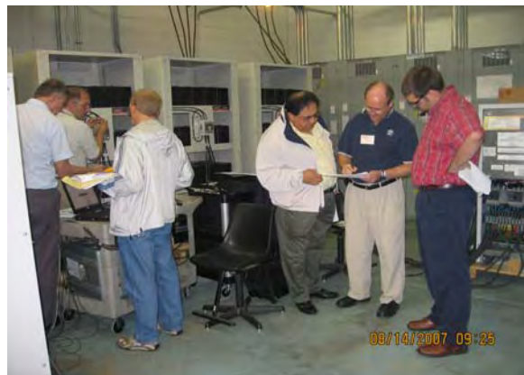
Factory Acceptance Testing of MSF/OCC Uninterruptible Power Supply Equipment
