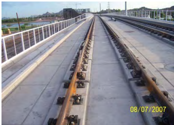
Track Expansion Joint on the South End of Tempe Town Lake Bridge
