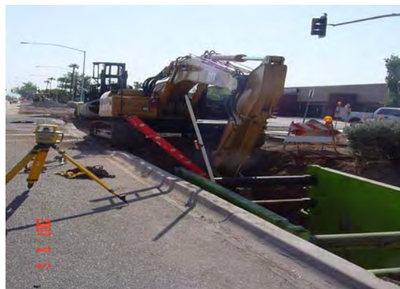
SRP irrigation installing new pipe at Ironwood along Main Street Road west of Sycamore in LS5
