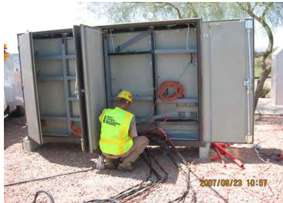
Washington Signal Case Terminating Cables at Signal Case
