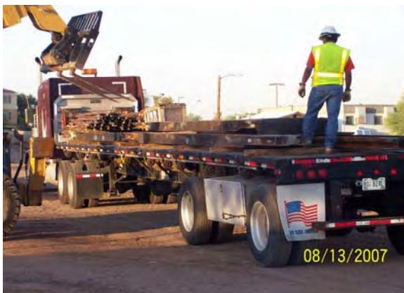
Delivery of two 100-Meter Crossovers to the Contractor's Storage Yard at LS5
