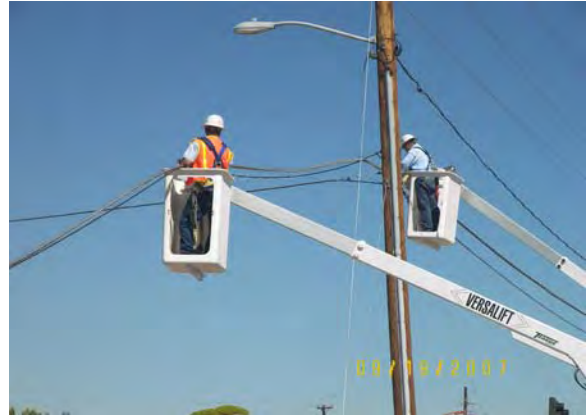
SRP power removing overhead electric and power poles on 19 th Avenue – north of Colter in LS1
