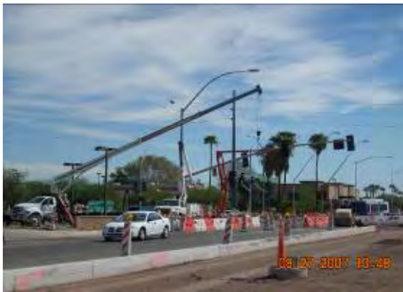
Replacement of Traffic Signal at Dobson/Main, Previously Removed to Facilitate SRP Work, Milestone E
