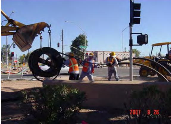
Qwest placing new 400 & 900 Pair cable – relocating due to SRP Irrigation conflict at Main Street and Sycamore in LS5
