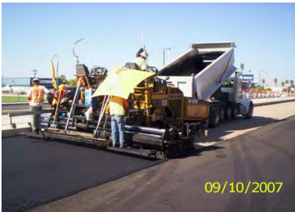
AC Paving - Crews placing AC on Camelback Road between 11th and 15 th Avenue
