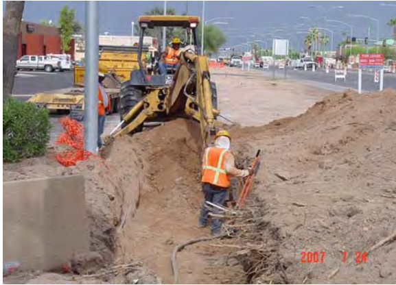
Qwest relocating cable in conflict with proposed SRP-Irrigation along Main Street in LS5
