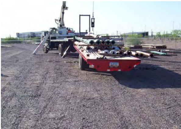
Traffic Signal Poles and Mast Arms being issued to the LS3 Contractor
