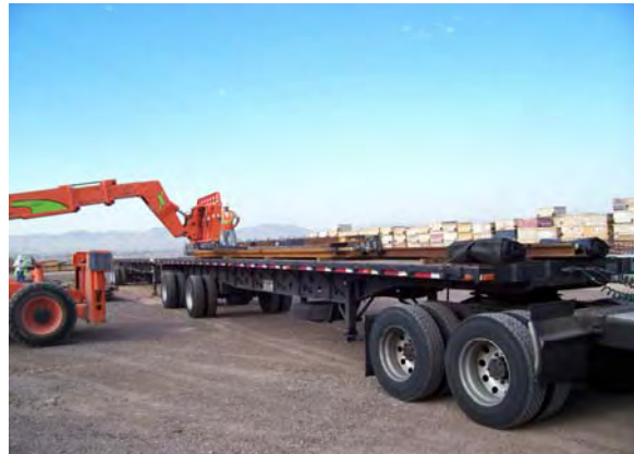
Delivery of two 100-Meter Crossovers to the Contractor's Storage Yard at LS2
