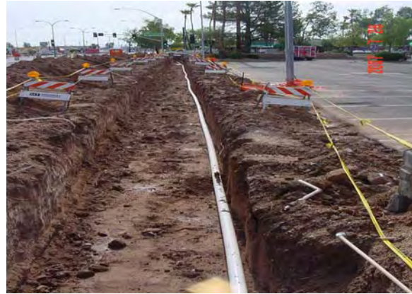
Qwest relocating conduit in conflict with proposed SRP-Irrigation along Main Street west of Sycamore in LS5
