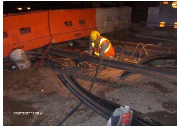
Grinding the welds at the Right track left and right rail at 15th Avenue
