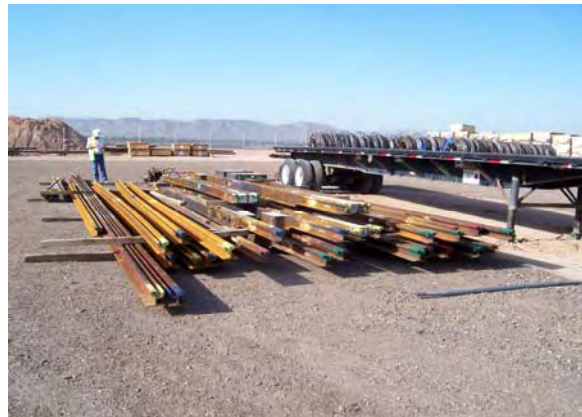
Delivery of two 100-Meter Crossovers to the Contractor's Storage Yard at LS2
