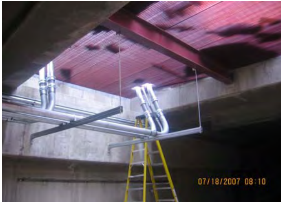
Signal Room Number 2 Installed Electrical Conduits
