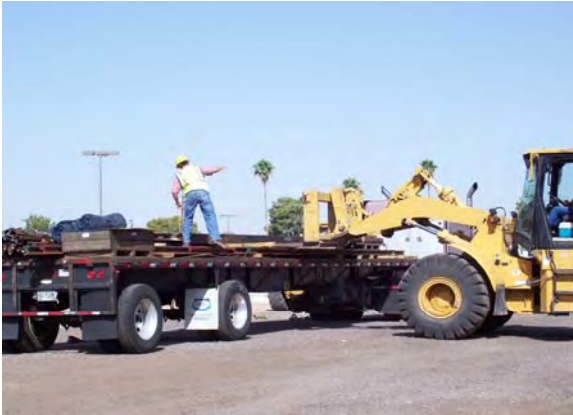
Delivery of a 100 Meter single crossover to the Contractor's rail yard at Line Section 1
