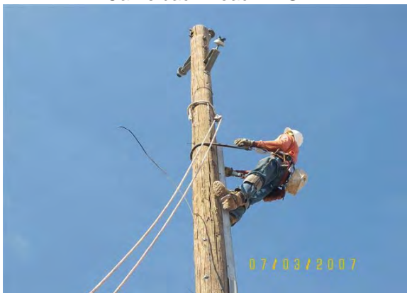
SRP Power removing overhead 12 kV along 19 th Avenue south of Camelback Road in LS1
