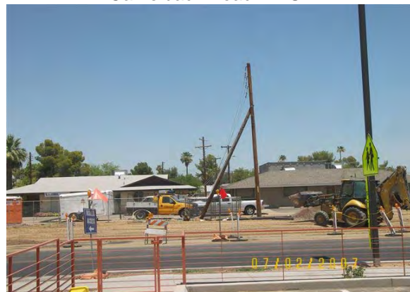
Qwest and Cox removing overhead cable on north side of Camelback Road in LS1
