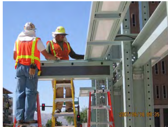
Mounting Station Visual Message Board
