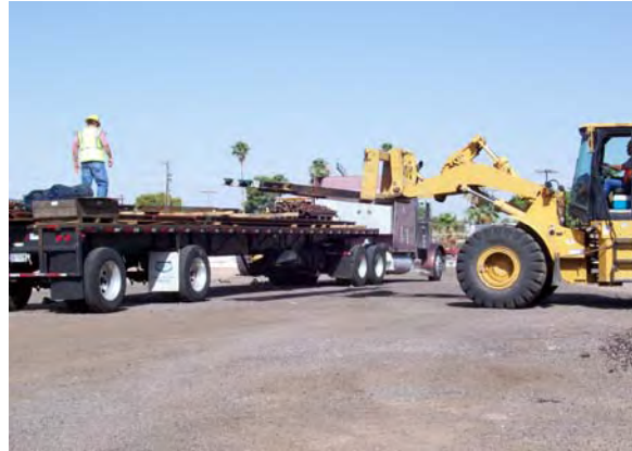
Delivery of a 100 Meter single crossover to the Contractor's rail yard at Line Section 1
