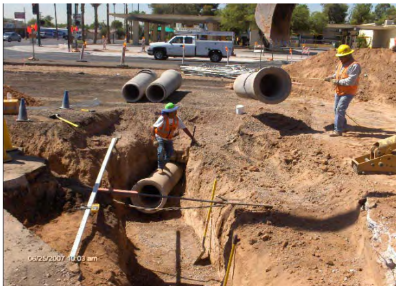
KWC crew installs new 18 inch RGRCP for the SD lateral at CBC15 425+18
