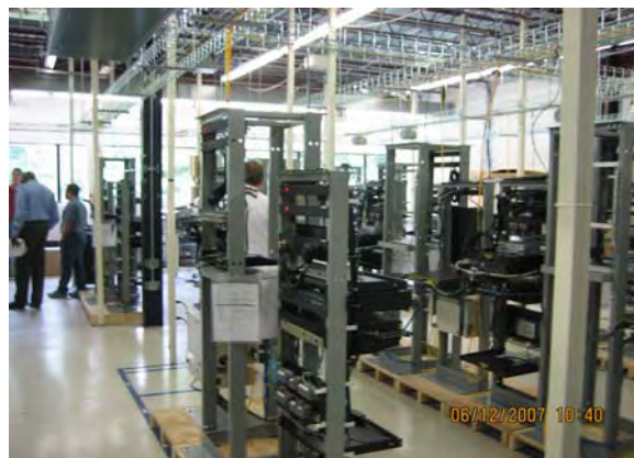
Performing Communications Factory Acceptance Testing of Rack Equipment
