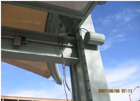
Station Public Address Speaker Installed
