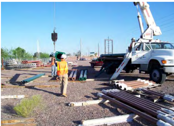
Traffic Signal Poles and Mast Arms being issued to the Line Section 3 Contractor
