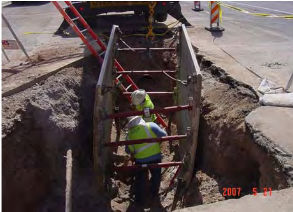
SRP Water installing irrigation pipe on Apache Boulevard from River to Price Freeway in LS5
