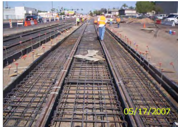
Guideway - P&CS crew performing the Holiday testing on the Rail Boot in the Guideway section from R Sta. 1077+35 to 1074+95, Rt and Lt track
