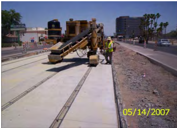
Guideway Curb - RGG crews preparing to place slip form Guideway Curb from R Sta. 1099+05 to 1099+75+/-
