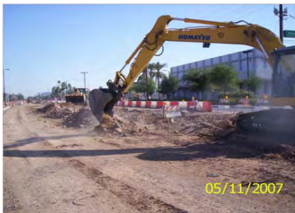
CTB Removal-KWC crews removing the CTB from Sta. 312+00 to 315+00 on 19th Avenue
