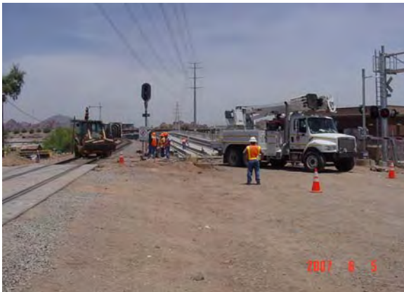
UPRR removing Signal Cabinet, Gate and Cantilever at 1 st Street and Ash in LS5
