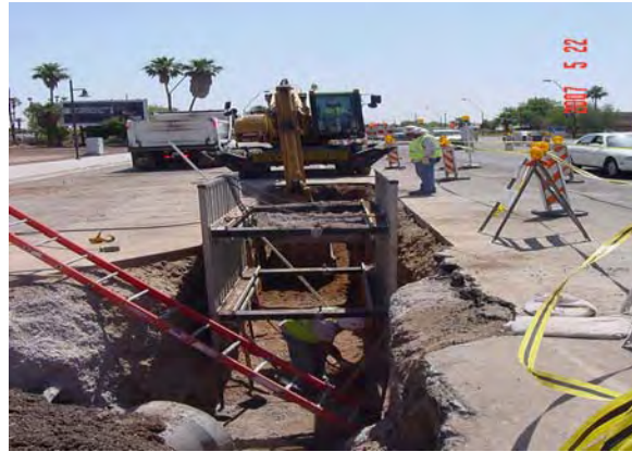
SRP Water installing irrigation structure Price Freeway and Apache Boulevard in LS5
