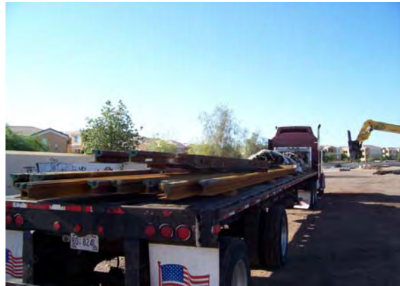
Delivery of a 100 Meter single crossover to the Contractor's rail yard at Line Section 5
