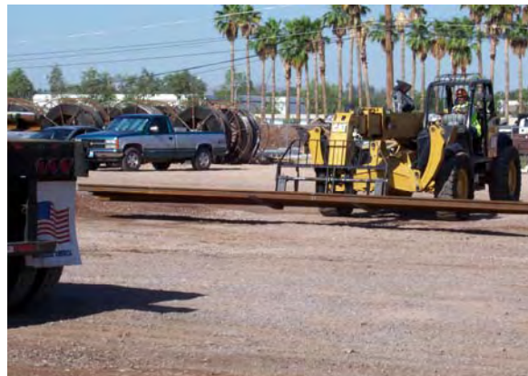
Delivery of a 100 Meter single crossover to the Contractor's Yard at Line Section 5
