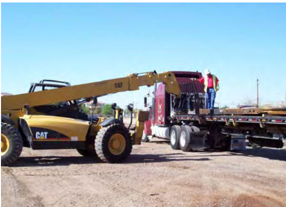
Delivery of a 100 Meter single crossover to the Contractor's Yard at Line Section 5
