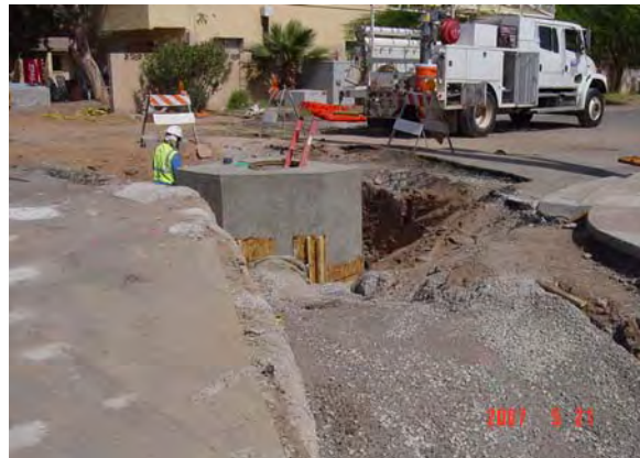
SRP Water setting a manhole at Rivers and Apache Boulevard in LS5
