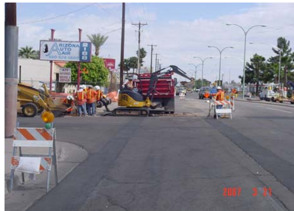
SRP Power - boring place conduits for 12 kV on Apache Boulevard in LS5
