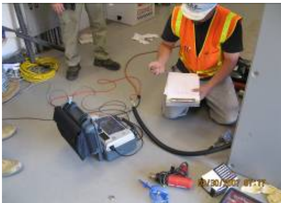
Hi-Pot Testing in TPSS No. 9
