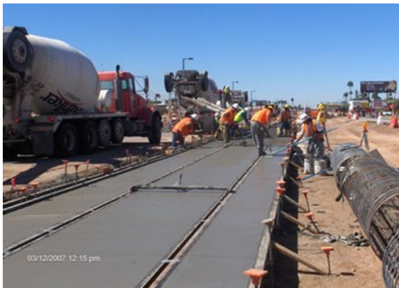
RGG placing and finishing the concrete for the Rt Track between 1096+20 and 1094+20.
