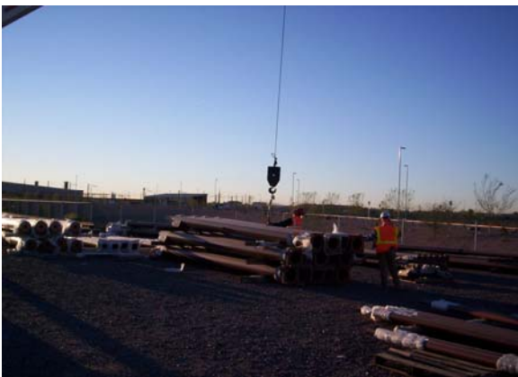
Contractor being issued traffic signal poles for Line Section 3 at METRO's Storage Yard
