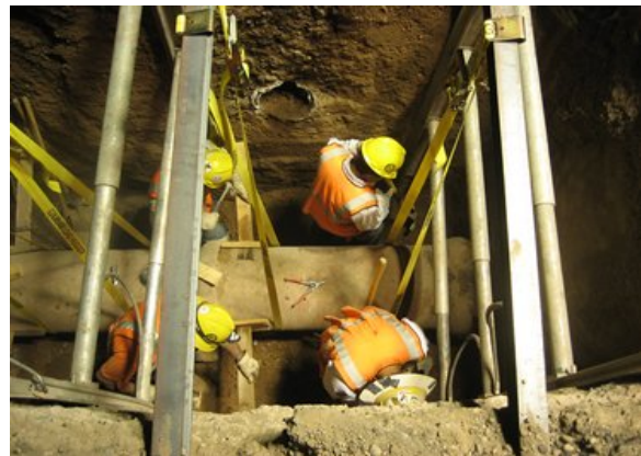
KWC Crew excavation of existing 18 inch sewer for casing Sta 453+10 North-South 7th Avenue.
