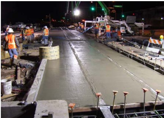
Placing concrete at LT guideway north of Campbell Station through Campbell Intersection
