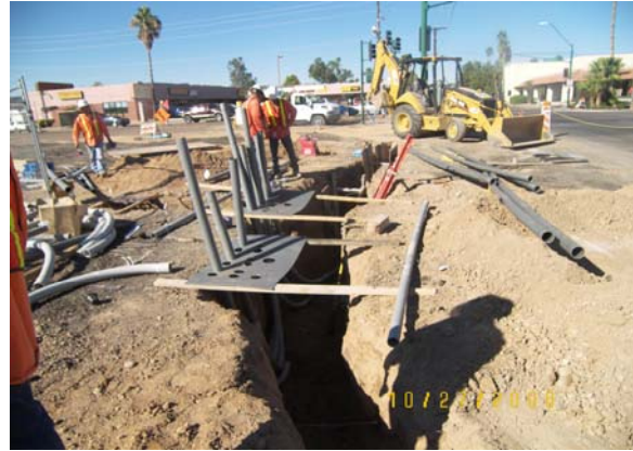
SRP-Power along Camelback Road in LS1
