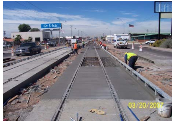
Guideway construction west of the Washington Street Bridge over the Grand Canal
