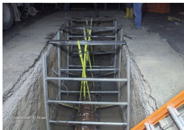
KWC crews placed concrete for the last 24 feet of 18 inch sewer for casing Sta 453+10.71.
