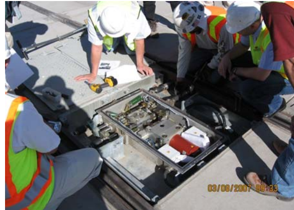
Yard Entrance - Switch Machine Adjustment Demonstration
