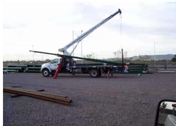
Contractor being issued traffic signal poles for Line Section 4 at METRO's Storage Yard
