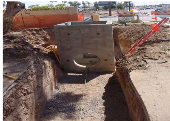
SRP Water – relocation irrigation pipes east and west of Rivers on Apache Boulevard in Line Section 5
