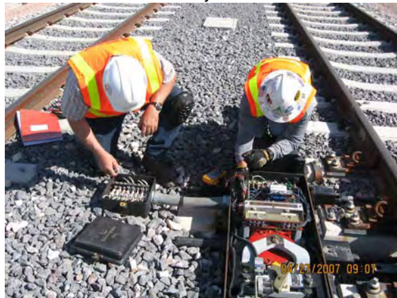
Yard Lead - Switch Machine Circuit Adjustment
