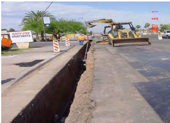
SWG lowering 600-feet of gas main on Apache Boulevard at Smith-Martin in Line Section 5
