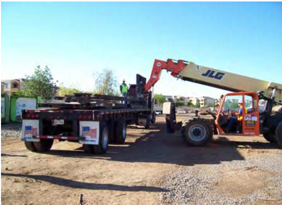
Delivery of a 100 Meter crossover to the Contractor's rail yard at Line Section 5
