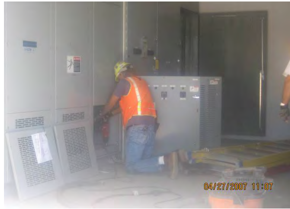
Anchoring of the TPSS Equipment at TPSS Number 5
