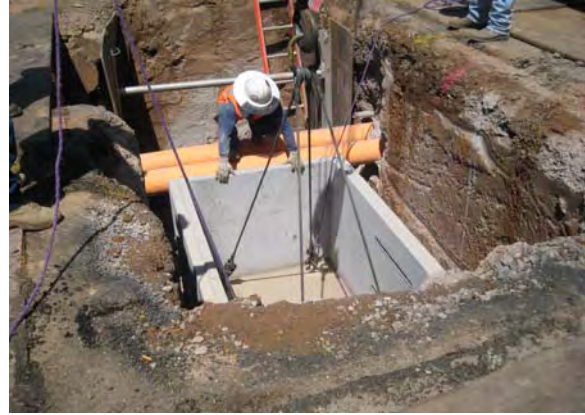
APS installing spare 230 kV pipes and manhole on Central Avenue and Encanto Boulevard in Line Section 2
