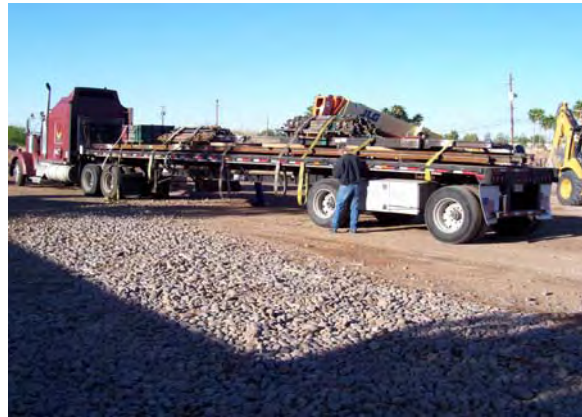
Delivery of a 100 Meter crossover to the Contractor's rail yard at Line Section 5
