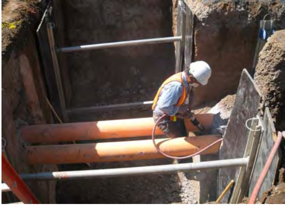
APS installing spare 230 kV pipes on Central Avenue and Encanto Boulevard in Line Section 2
