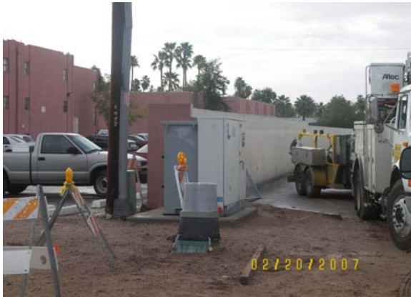
SRP-Power relocation at the Fry's property along Camelback Road in Line Section 1
