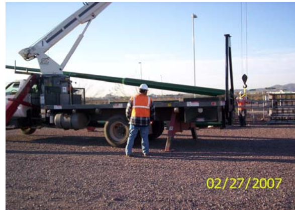
Contractor being issued traffic signal poles for Line Section 4 at METRO's Storage Yard.
