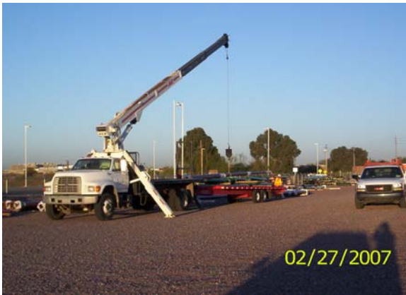
Contractor being issued traffic signal poles for Line Section 3 at METRO's Storage Yard.
