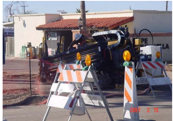
SRP Power - boring place conduits for 12 kV on Apache Boulevard in Line Section 5
