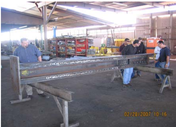
Station Shade Structure - Steel Fabrication at Skyline Steel, Gilbert, AZ (Archer Western Subcontractor and steel installer)
