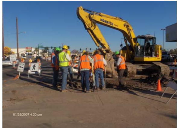
KWC Staff Working on locating water 2 inch water service corp stop to shut water off for the service that was hit by KWC removal crew at 396+80 Camelback
