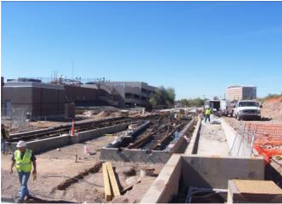
Switch Placement, East Bathtub
