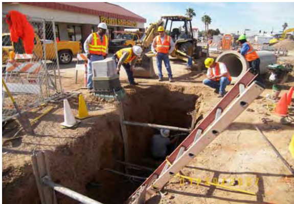
SWG relocation at the Fry's property on Camelback Road in Line Section 1
