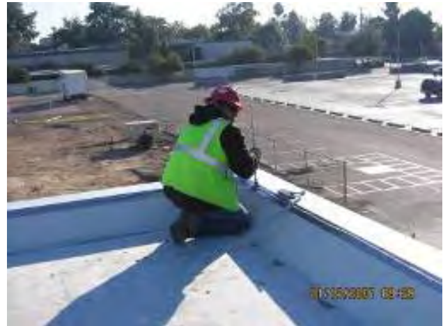
TPSS No. 1 - Lightning Protection Installation
