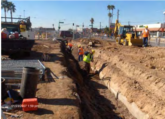
KWC placing the top lift of bedding over the new 12 inch DIP water line between 415+50 and 416+50
