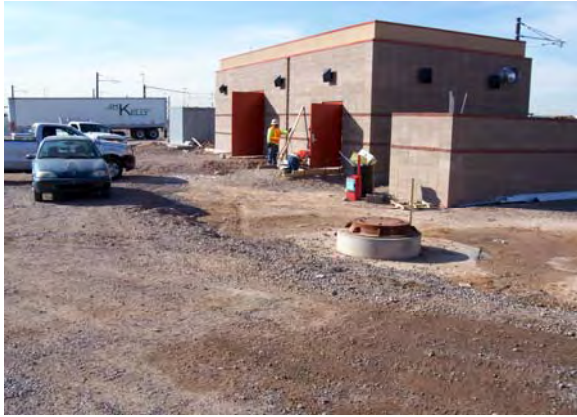
Traction Power Substation No. 15
