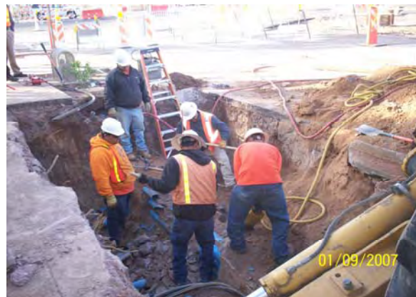
Qwest Fiber Optic duct bank damaged and repair, North of Highland
