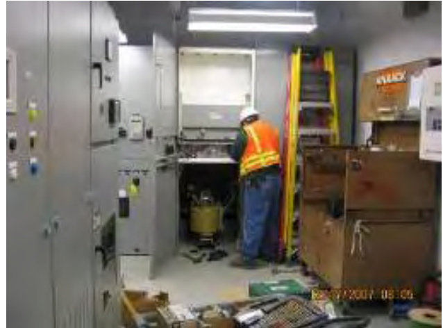
TPSS No. 9 – AC Compartment Wiring
