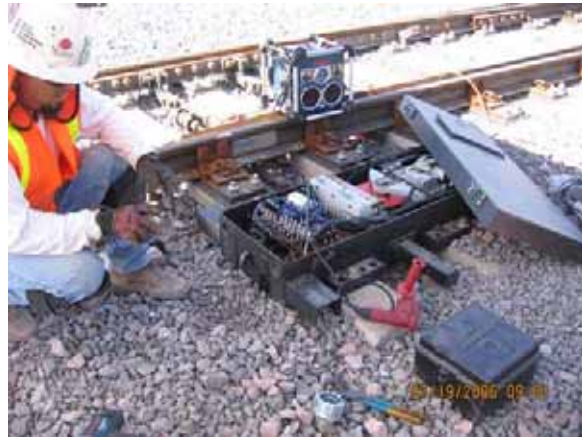
MSF Yard - Wiring Switch Machine Terminations
