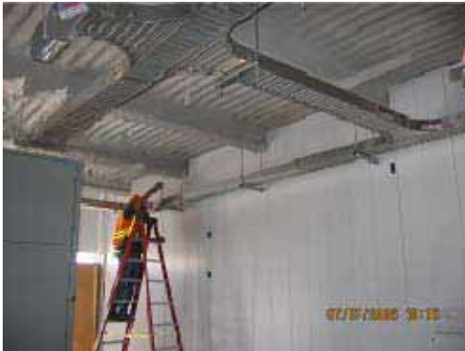
Cable Trays at TPSS No. 9
