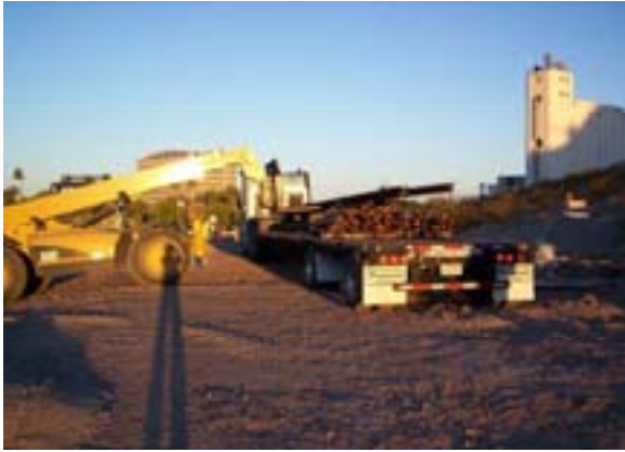
Early morning delivery of the embedded pocket track material for Line Section 5
