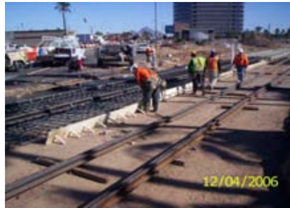
12-04-06 Guideway - RGG crews forming the Guideway section E-2 at R Sta. 1103+50, Lt. track Central to the 3rd Ave
