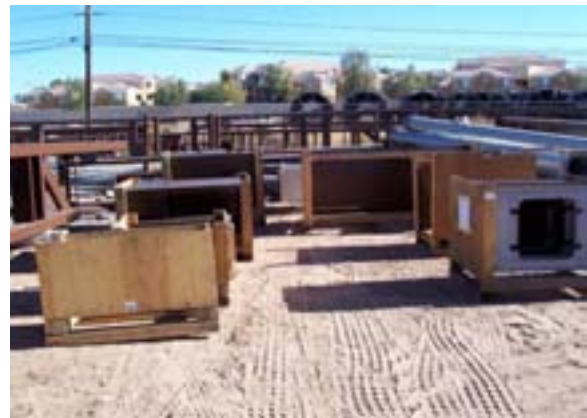
Delivery of blank out panels for Line Section 4 and 5 traffic signal structures
