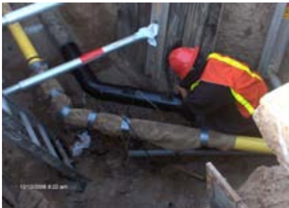
12-12-06 SWG Tie-In- Installing Cathodic Protection for the new gas main at 19th Ave.
