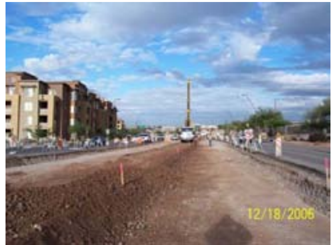
Rough grading for guide-way and OCS foundation drilling east of Center Parkway
