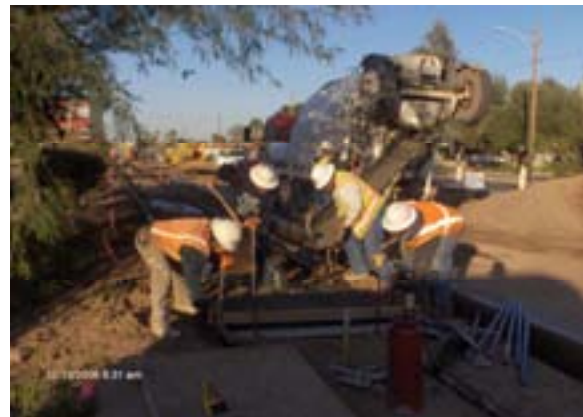
12-13-06 5ft Sidewalk- CPI placing 2500psi concrete for the sidewalk between station 439+00 to 437+00 between 11th and 13th Aves.
