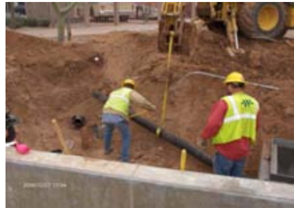
Drainage features between Van Buren and 1 st Avenue and Central Avenue Couplet Stations in Downtown Phoenix
