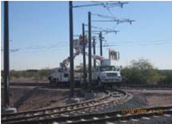
OCS Adjustments for the Storage Lead Wire Run
