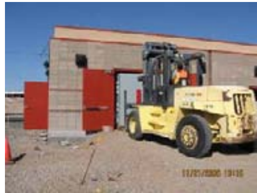
TPSS No. 15 Equipment Delivery
