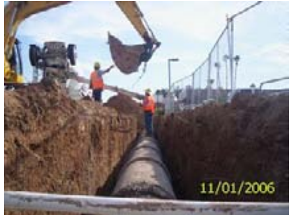
11-01-06 KWC Crews Installing The 24 Inch SRP Irrigation Line At 19th And Colter.
