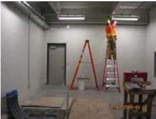
Cable Tray Supports at TPSS No. 16
