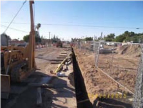
SWG 4-inch High Pressure main on 19 th Avenue in Line Section 1
