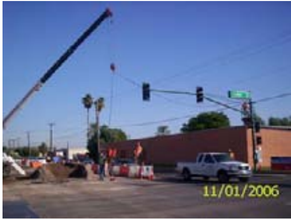
11-01-06 CW Crews Stringing The Temporary OE At 19th And Colter For The Traffic Signals
