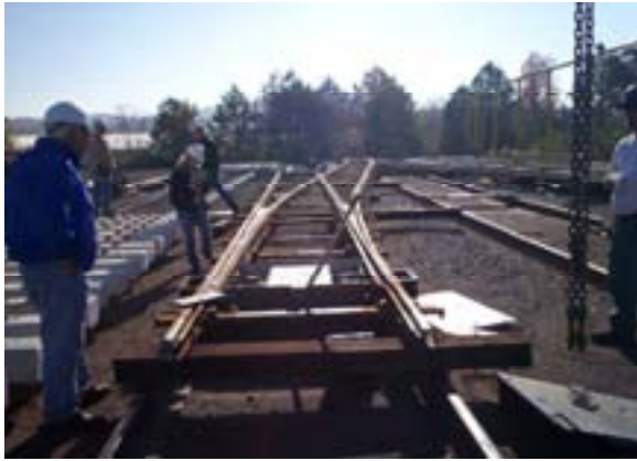
First Article Inspection of the LS2 Single Crossover
