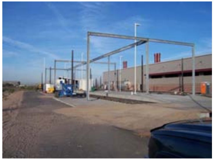
Sand distribution system supports at the Yard Service and Cleaning Platform
