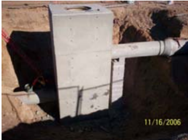
SRP Irrigation manhole and piping
