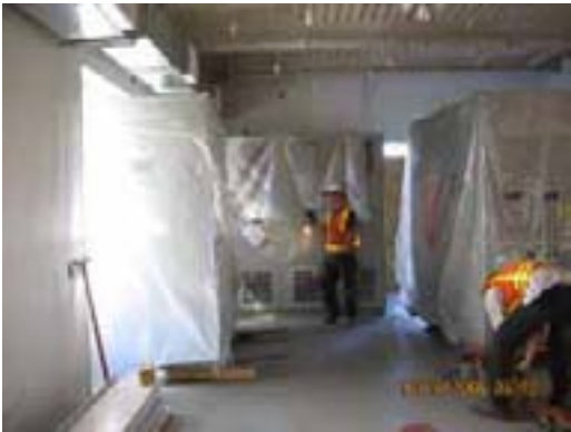
TPSS Equipment at TPSS No. 6
