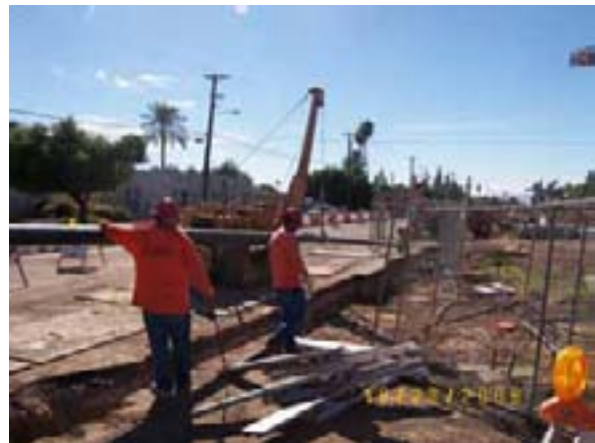
SWG relocation 8-inch High Pressure Gas Main on 19 th Avenue in Line Section 1
