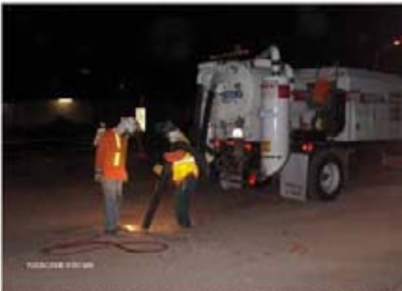
HMS Potholing to locate existing utilities from 13 th Avenue to 15 th Avenue at the south side of the road for the new 12-inch waterline work
