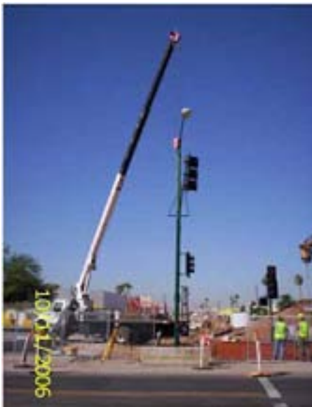
KWC requested that CW support the existing TS pole at the southwest corner of 15th Avenue and Camelback Road while installing SRP Irrigation Lat.
