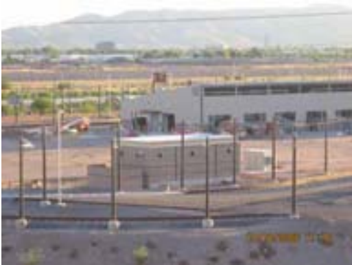
Overview of the MSF Yard OCS Installation
