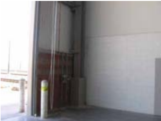
Switch Installed for Temporoary DC Power Distribution in the MOE
