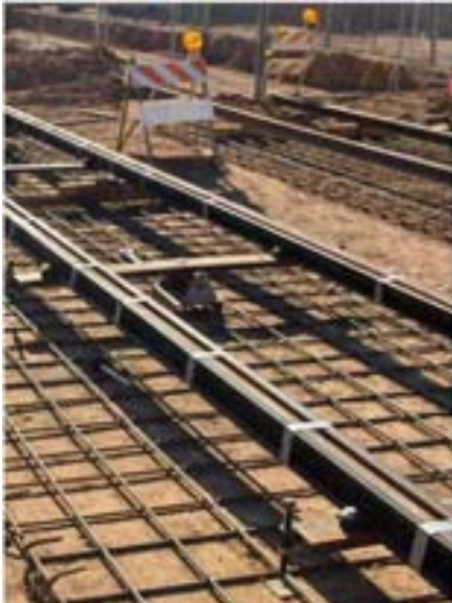
KWC have set line, grade, guage and X-level to final from STA. 1106+00 to STA. 1104+75 004
