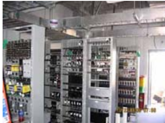
SB No. 4 - Installed Signal Racks
