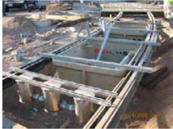
Yard Entrance - Mounted Signal Cans and Impedence Bond Earth Boxes
