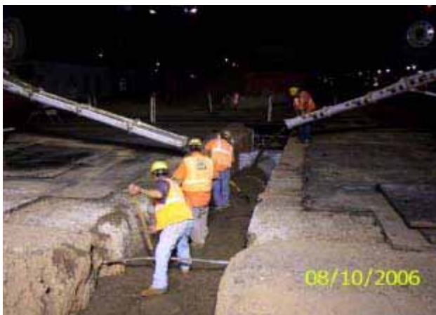
KWC crews placing slurry on the 30-inch SRP Irrigation line at STA. 453+40
