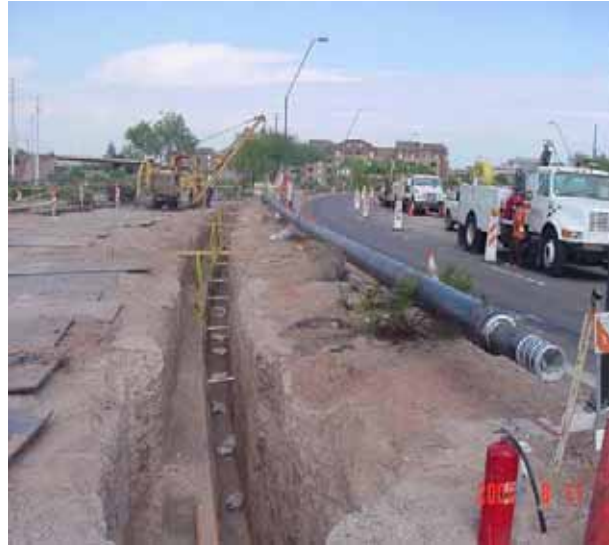
SWG relocation 8-inch High Pressure Gas Main on Washington Street and Lakeview Drive in Line Section 4
