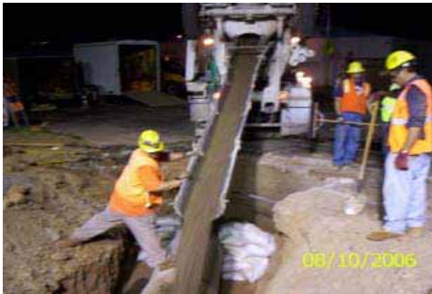
KWC crews placing slurry on the installed 24-inch private irrigation line at STA. 453+60
