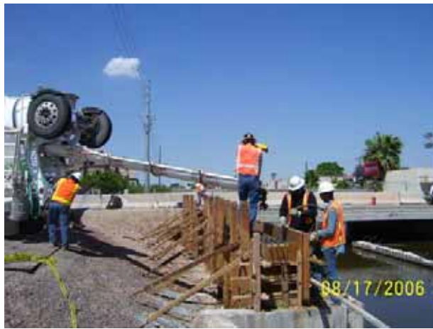
Pouring Grand Canal Bridge abutment on the south end of the bridge.
