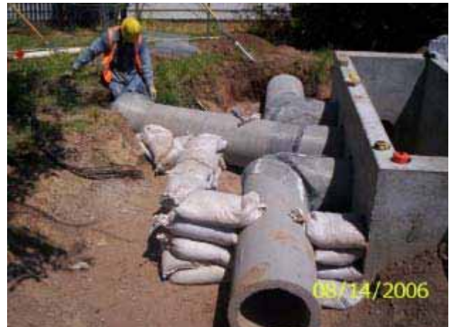
KWC crews preparing pipe collars for the private irrigation line connection at STA. 330+ on 19 th Avenue
