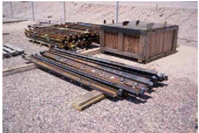
Crossties for Turnout 3-5 and 3-6 that is to be installed on Line Section 3.
