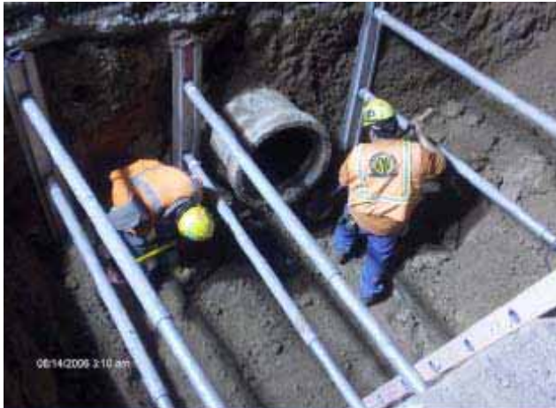
KWC hand digging around the existing 21-inch CP in preparation to install the new SRP manhole number seven
