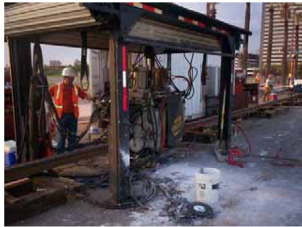
Ribbon Weld flash butt welding rail into strings near Steele/Indian School Park.
