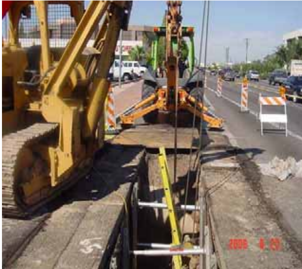
SWG relocation 8-inch High Pressure Gas main at 19th Avenue & Camelback Road in Line Section 1
