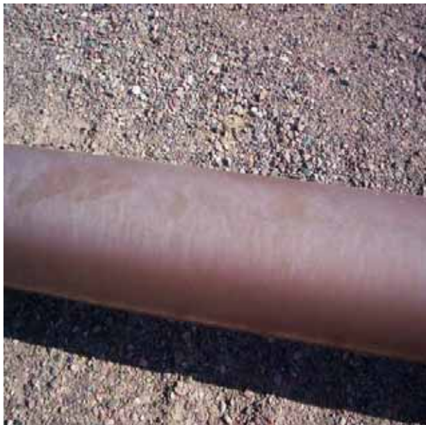
Copper colored poles have developed an oxidation problem
