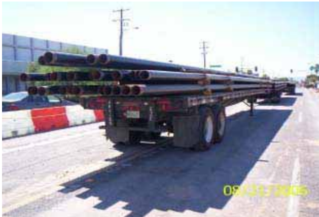
Stockpiled 6-inch steel gas line on 19 th Avenue between west and east Montebello Roads
