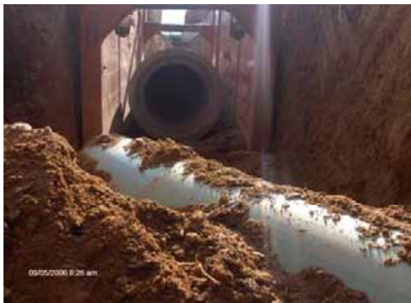
Fry's Parking Lot Storm Drain in Conflict with the New SRP at 415+87
