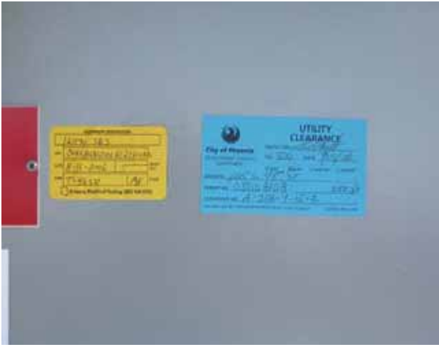
Utility Clearance – City of Phoenix Blue Tag
