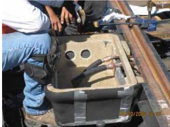
Yard Entrance - Rail Bonding Shunt Fouling Pigtails
