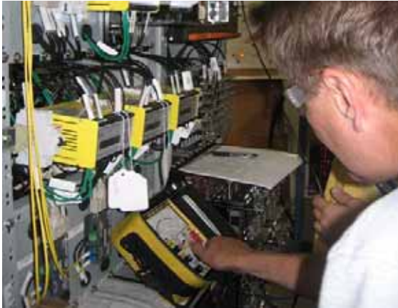
FAT Culver Interlocking Signal Equipment
