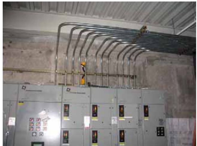
Motor Control Center for the LRV Lift
