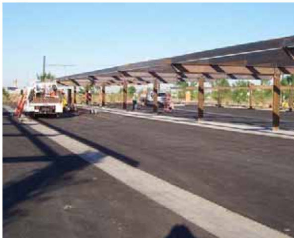
Shade Canopies in the MOE Parking Lot
