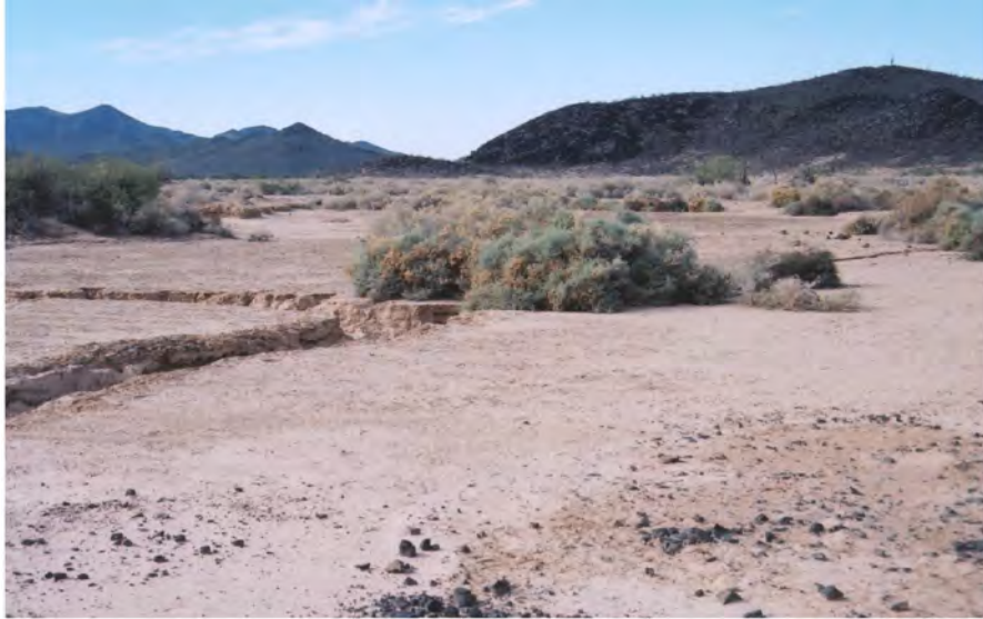
Figure 7. Intersection of cracks near northwestern end of main cluster, Winter 2002.
