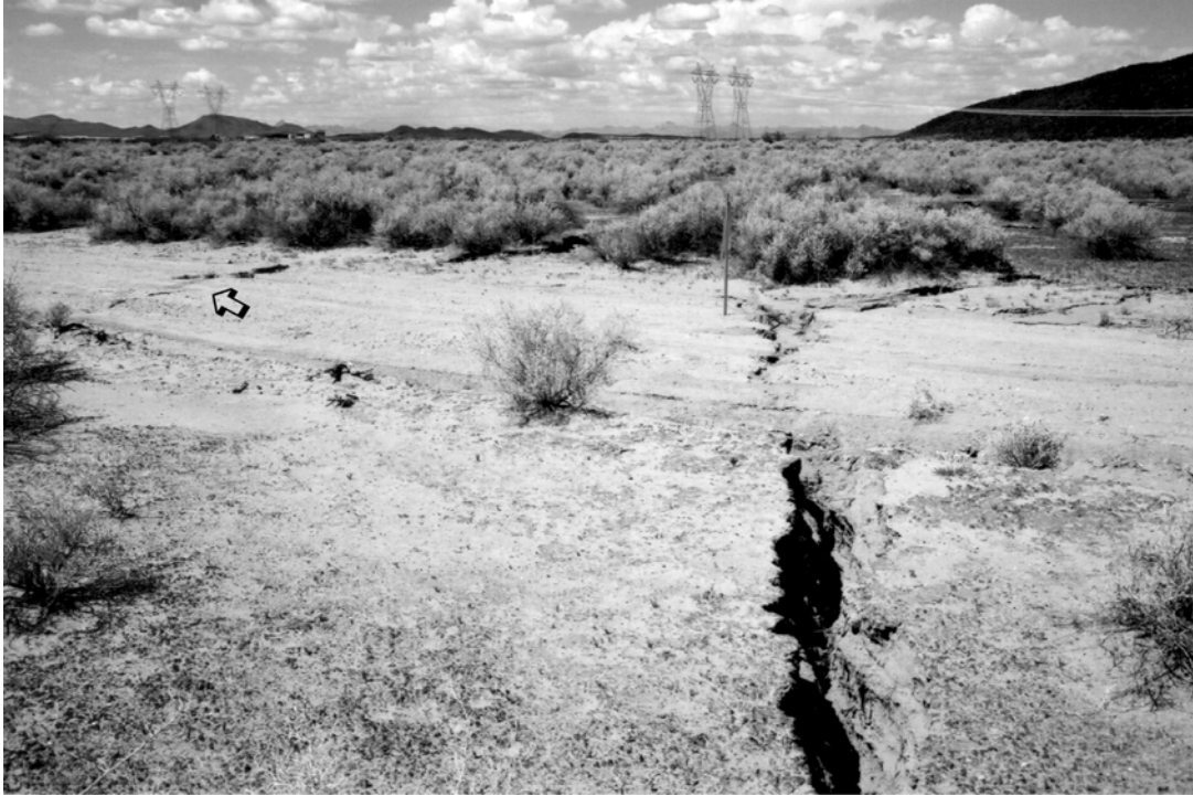
Figure 5. En echelon section of earth fissure crossing Baseline Road, looking NW. Fissure is 6-12 inches wide here. Second earth fissure crosses road at far left (arrow).
