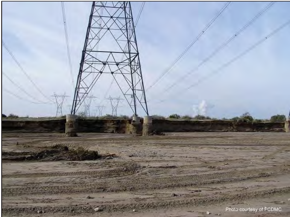
Lateral bank migration at SRP poles
