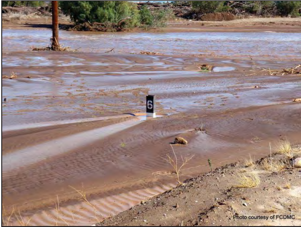
Sediment deposition at Tonopah Salome Highway
