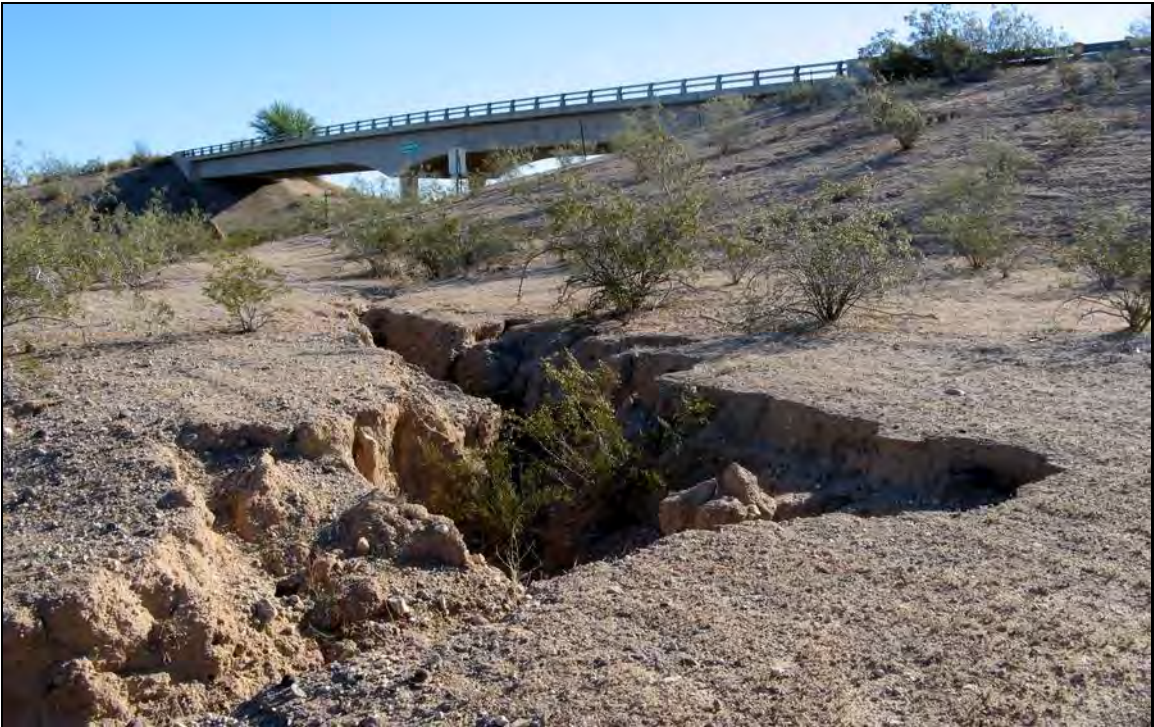
644: Erosion SE of Johnson Rd crossing of I-10
