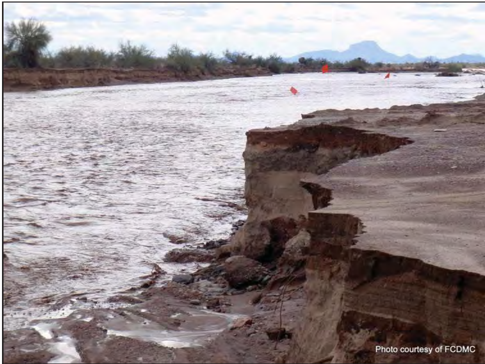
Bank erosion at Tonopah Salome Highway
