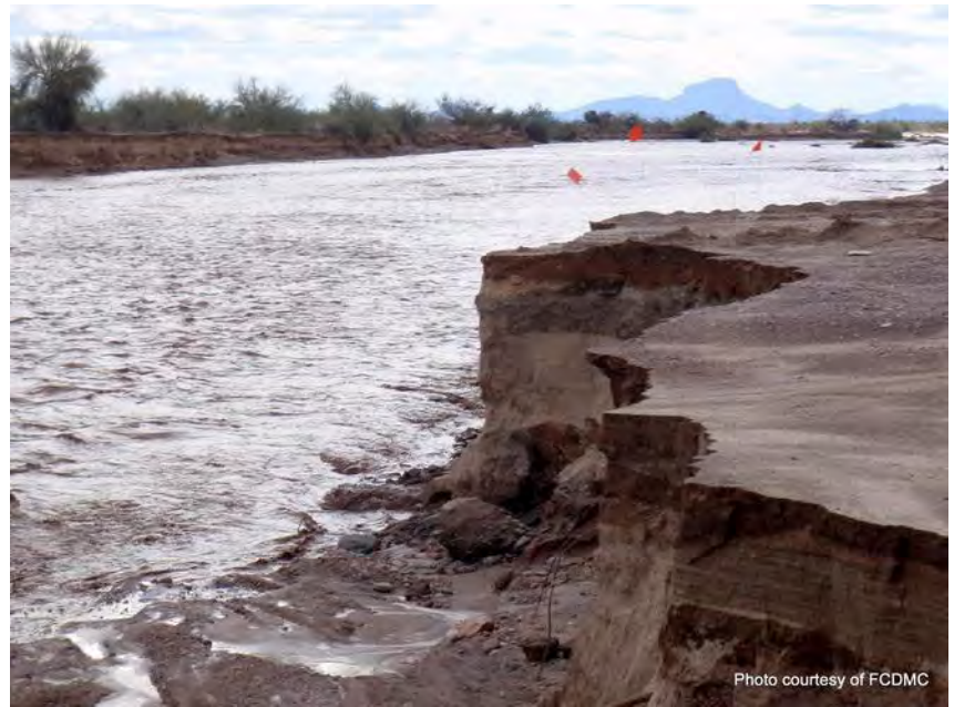
Bank erosion at Tonopah Salome Highway
