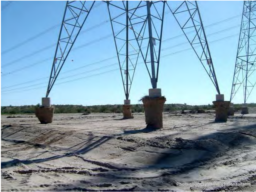
Channel erosion at SRP poles
