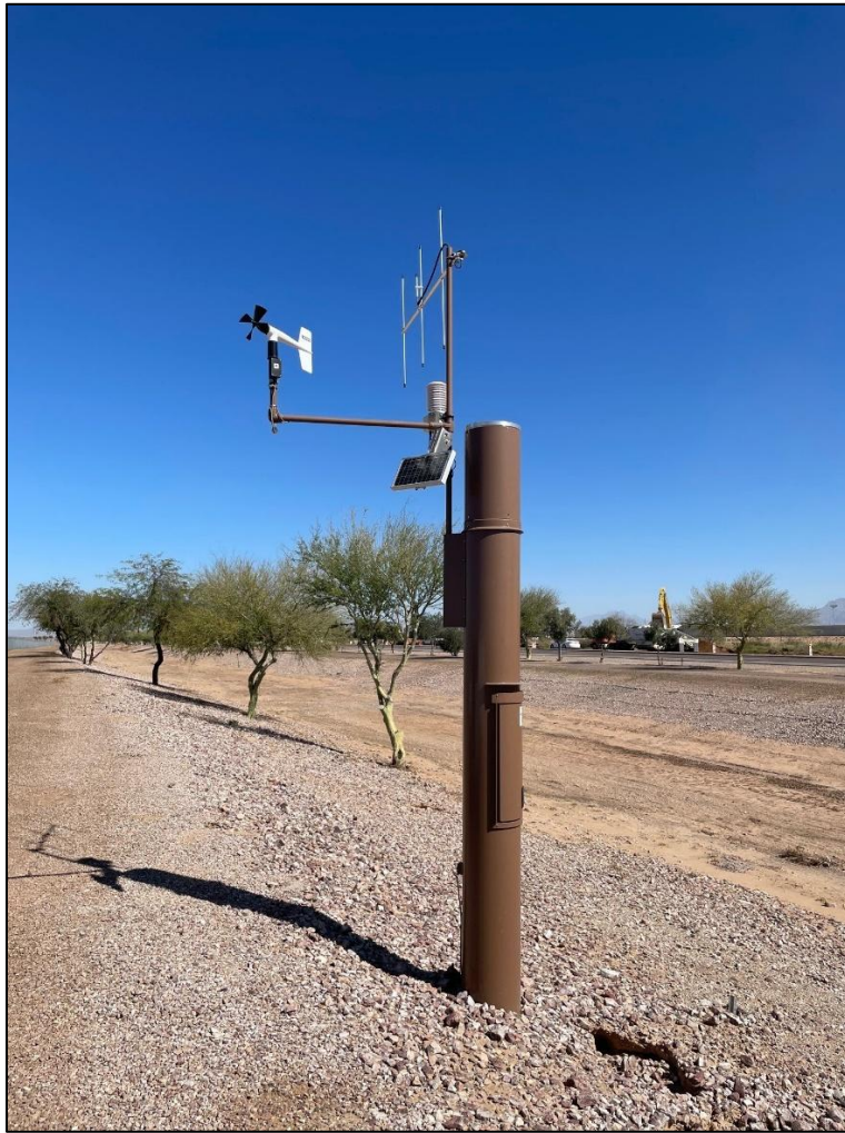
'Ellsworth Channel DPC' Rain Gage, Station # 50901, Installed 12/17/2024
