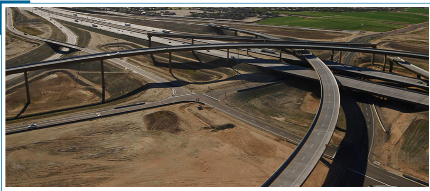
Aerial view of the I-10 and Loop 303 interchange during construction. The freeway has since been built to Van Buren Street, with plans underway to extend the Loop 303 to MC 85 by 2028.
