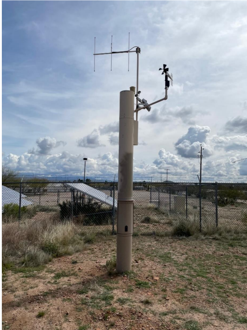
Wickenburg Weather Station
