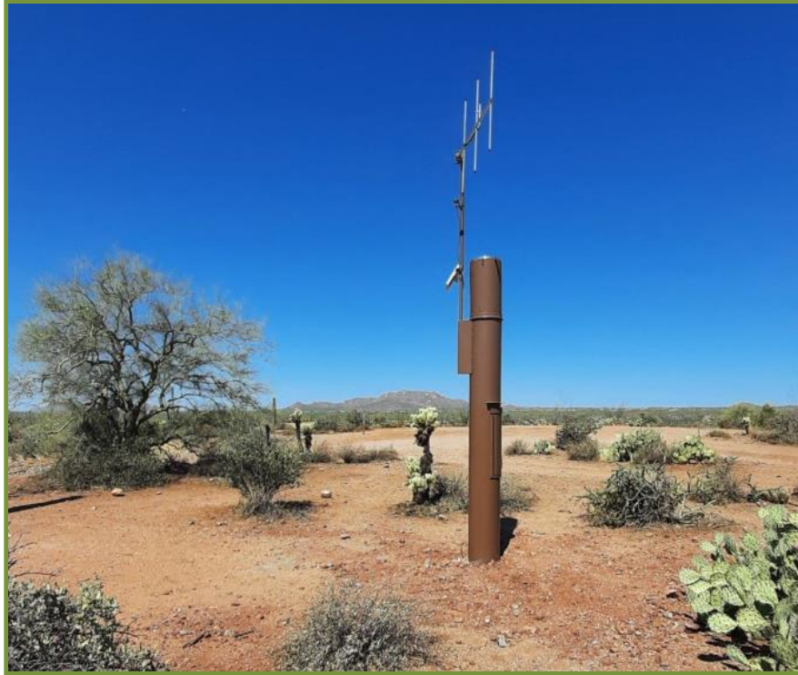
'Camp Creek Overlook' Rain Gage, Station # 50768, Installed 06/29/2022
