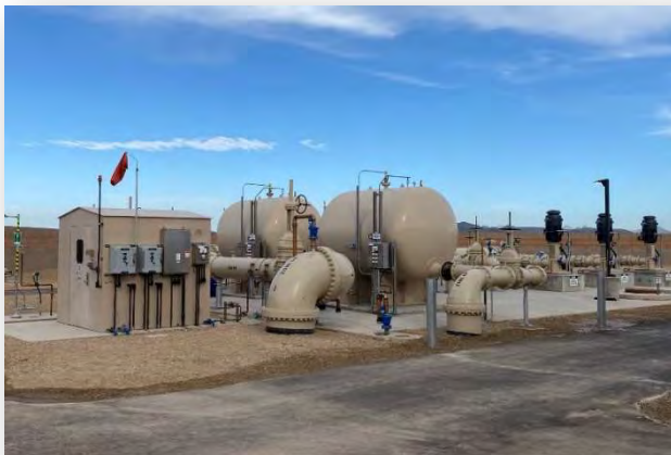
The Agua Fria Booster Station was financed with development impact fees
