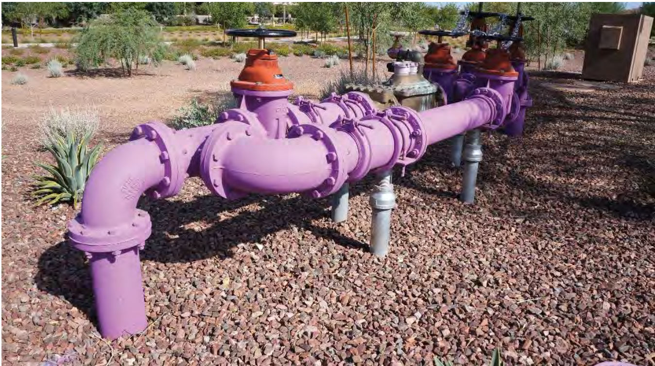
Purple Reclaimed Water Pipe
