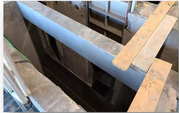
The Butler WRF Headworks were rehabilitated to correct extensive damage to the concrete surfaces
