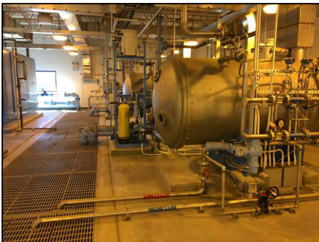
Greenway Water Treatment Plant
