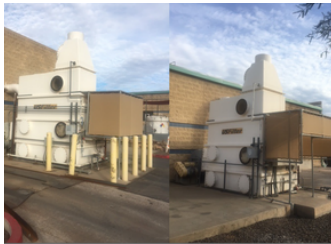
WRF Air Scrubbers
