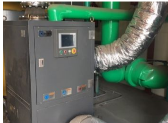
WW Process Equipment
