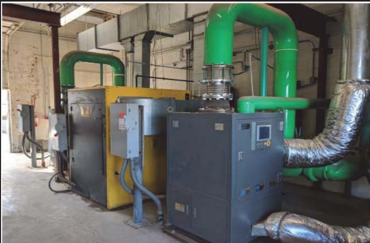
Current WRF Blower System
