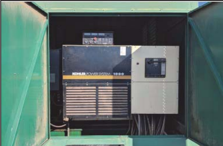
Existing WRF Diesel Genset
