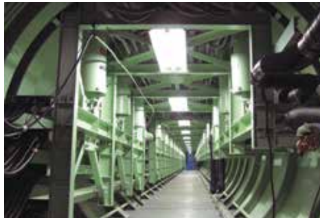
Long Cableway inside the Titan Missile site. Photo courtesy of the Titan Missile Museum
